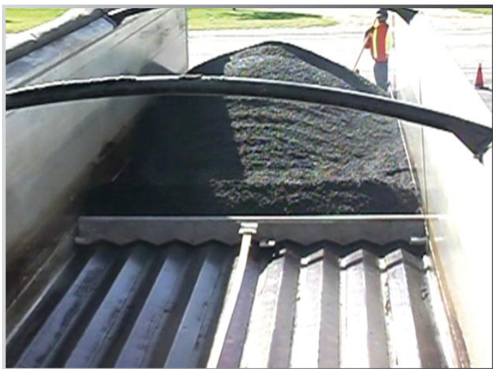
Titan's V-Plow system automatically cleans up the solid steel floor as the asphalt is walked off into the paver.
