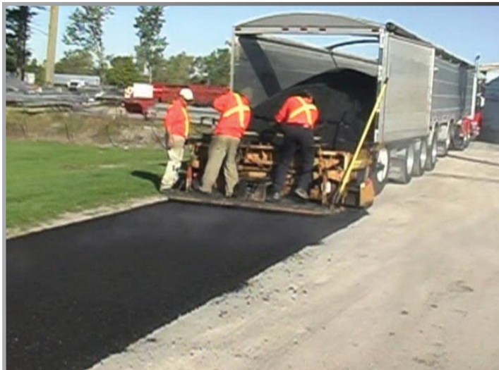
Keeping the trailer level as it unloads eliminates segregation of the material, so there's no need to remix before paving.
